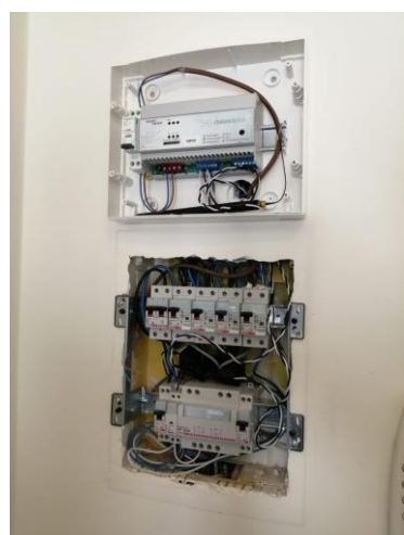
Figure 3-10 Power meter setup in the residential buildings (Monaci)
