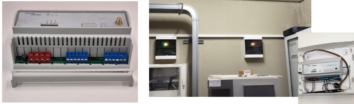
Figure 3-8 Smart power meter setup in the office buildings (Cubo #B)
